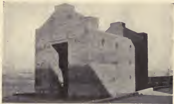
Shows completed walls ready for roof and finishing coat of plaster EARTH HOUSE, ST. LOUIS, MO. THOMAS CRANE YOUNG, ARCHITECT
